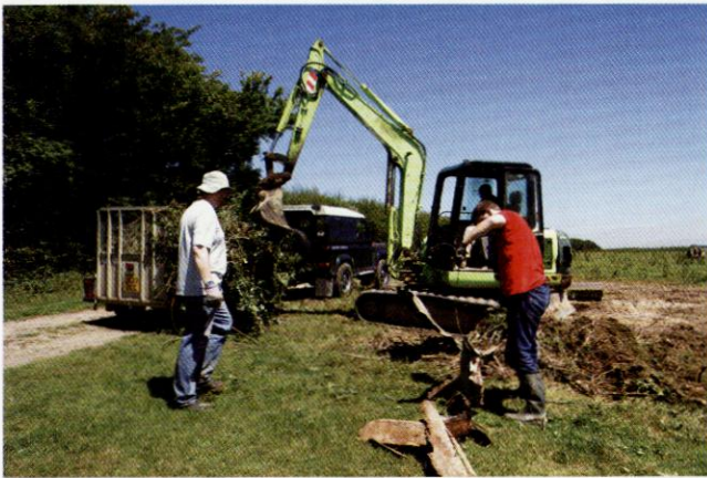
Nick and Dom Jackson help David (in digger) to clear the slab and cut the surrounding earth down to a level where it won't run off into the bunker.
